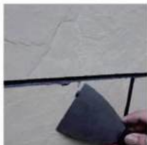
7. Use a hook to scrape off the areas contaminated by adhesive and cement slurry
