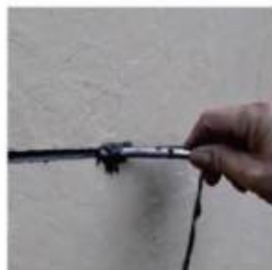
6. When the grout is half dry, use a steel bar to pull the seam
