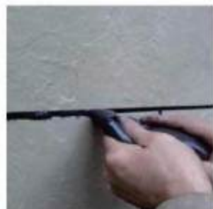
5. Use a plastic bag to fill the gap with grout or fill the gap with neutral silicone glue
