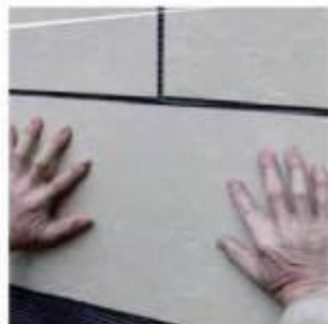
4. Move up and down to adjust the width of the space, and use a large board to compact the product to the wall
